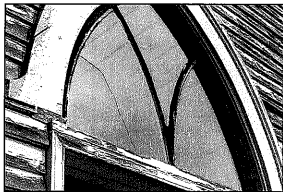
Figure 19: Cracked glass above entrance doors
