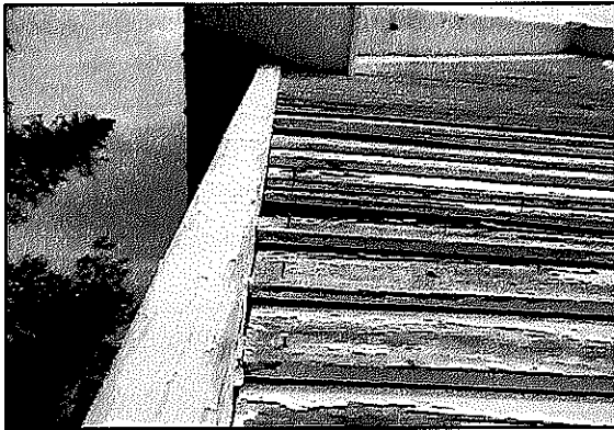
Figure 16: Cupping clapboards and popping nails on southwest corner of structure
